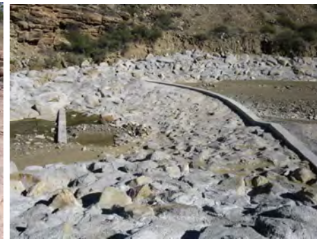
Grouted rip-rap (wire-enclosed or loose rock) - Above example is grouted loose rock. Average size of rock shown here is between 24 to 36 inches. Location is an arroyo paralleling NM 51, upstream of Elephant Butte Reservoir, Sierra County.
