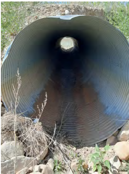
Minor corrosion on inside
