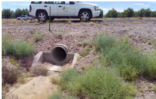
Culvert outlet shows little to no scour (less than 1 ft. depth). If outlet is covered partly in sediment, leave it as blank in data collector and move on. Location above is on NB I-25, south of Belen, Valencia County.
