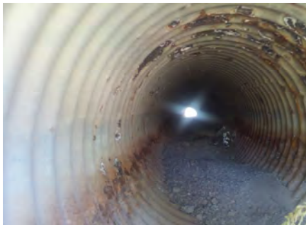
Major corrosion - metal is corroded through culvert on the top of culvert exposing the fill dirt surrounding culvert. Location is on US 60, Mountainair, Torrance County.
