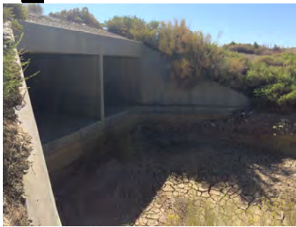
Major scour (from 3 ft. to 8 ft.) at the outlet of 2 barrel CBC. Note the absence of concrete apron, characteristic of older CBCs. Location Unknown.
