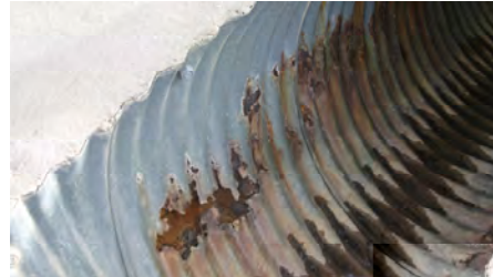
Major, metal has been corroded through culvert, exposing the fill dirt surrounding culvert. Location is WB I-25 MP 120.9.
