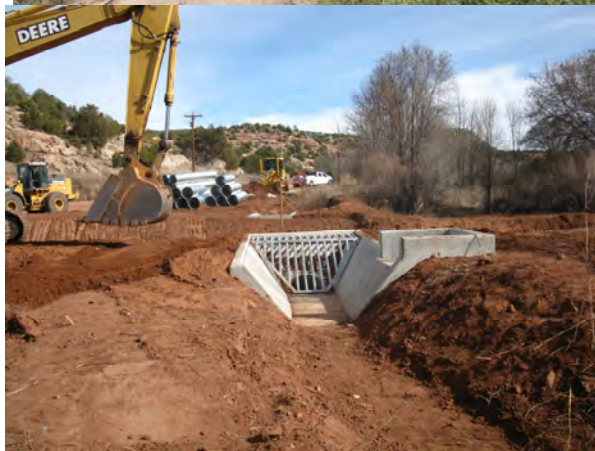
Concrete siphon used for irrigation ditches. Sample to the left has trash rack and built-in side gate. NM 3 near La Fragua, San Miguel County
