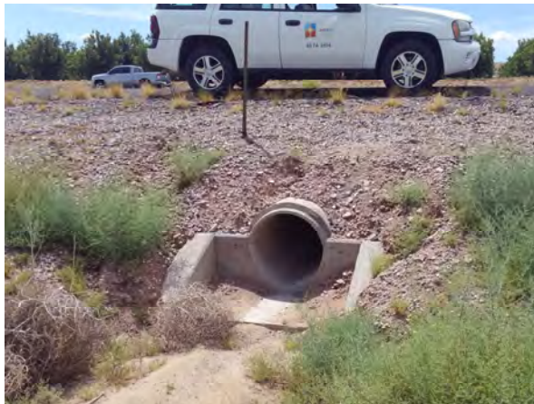
Concrete end sections common in construction of Interstates in the 1970s. Culvert to left is on I-25, south of Belen, Valencia County.
