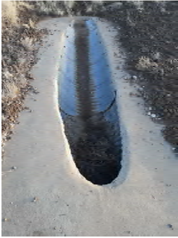
Metal culvert, no safety grate. Location is unknown.
