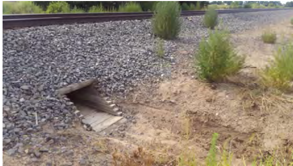
Location of timber box culvert shown on left is adjacent to NM 116, Jarales, Valencia County
