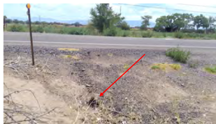
Greater than 90% silting. The culvert shown by red arrow is almost covered. Only the t-post to the left gives away the culvert's location.
