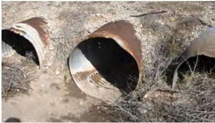
Major, corrosion on inside and outside. Location is on NM 2, north of Dexter, Chaves County.
