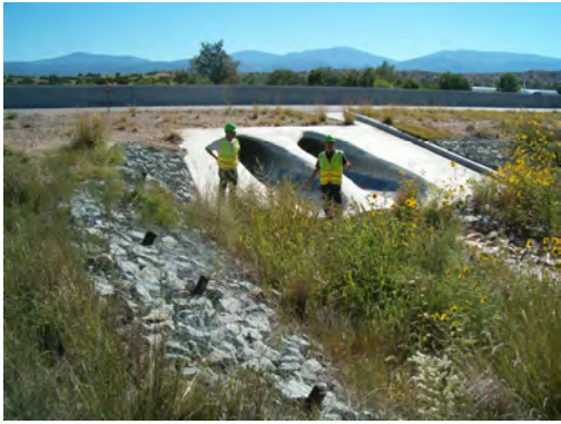
Concrete culvert pipe, no safety grate. Location is on US 84/ 285 south of Cuyamungue, Santa Fe County.
