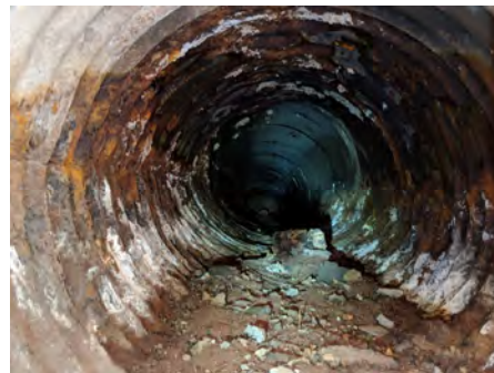
Major corrosion - metal is almost completely disintegrated. Location unknown.
