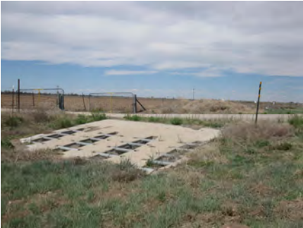
Metal culverts, with safety grates. Location is on NM 2 south of NM 438, Eddy County.
