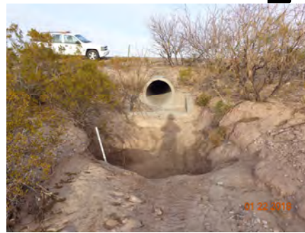
Major scour at the outlet of concrete culvert. Although a scour hole formed at the base of culvert, the surrounding soils are cohesive enough to resist further erosion of flowing water after losing its energy in the scour hole. Location above is on SB I-25 near Hatch, Doña Ana County
