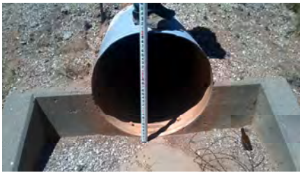
Minor corrosion on inside
