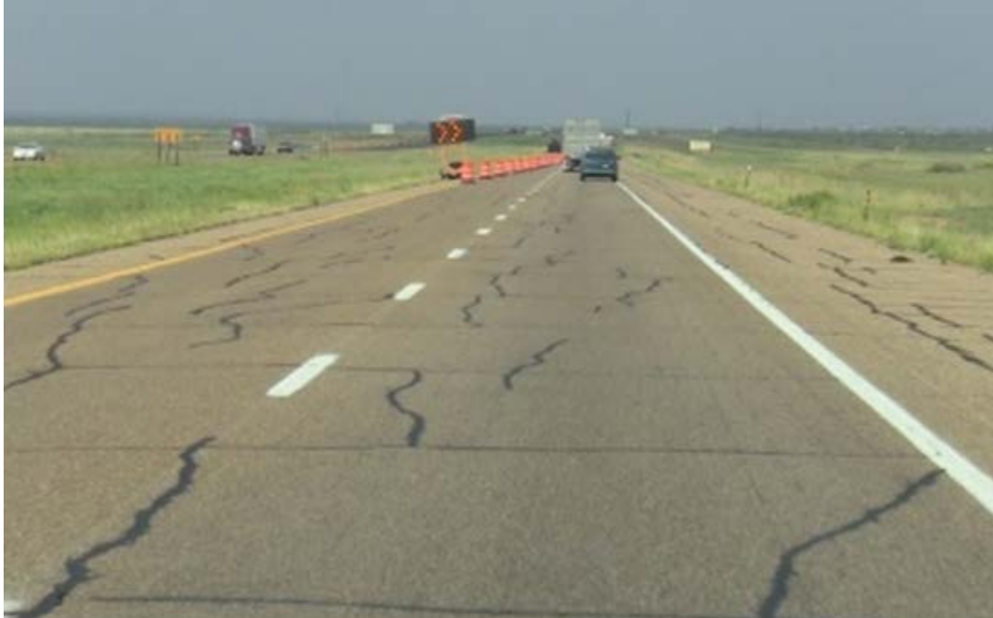
FIGURE 36 Road Condition before WMA Project.
