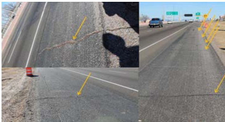
(b) Transverse Cracking on Shoulders
