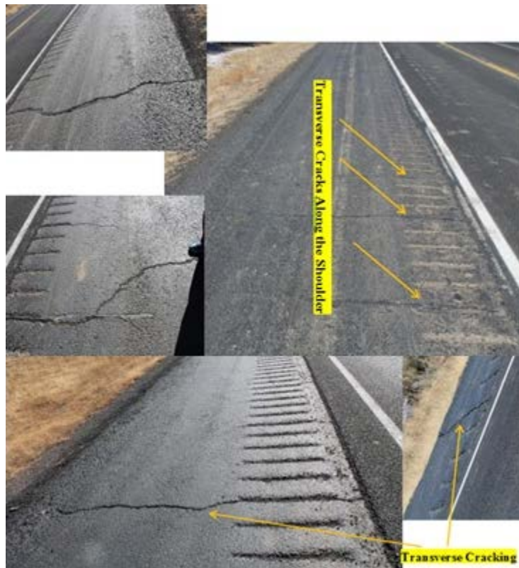
FIGURE 31 Transverse Cracking on Shoulders.
