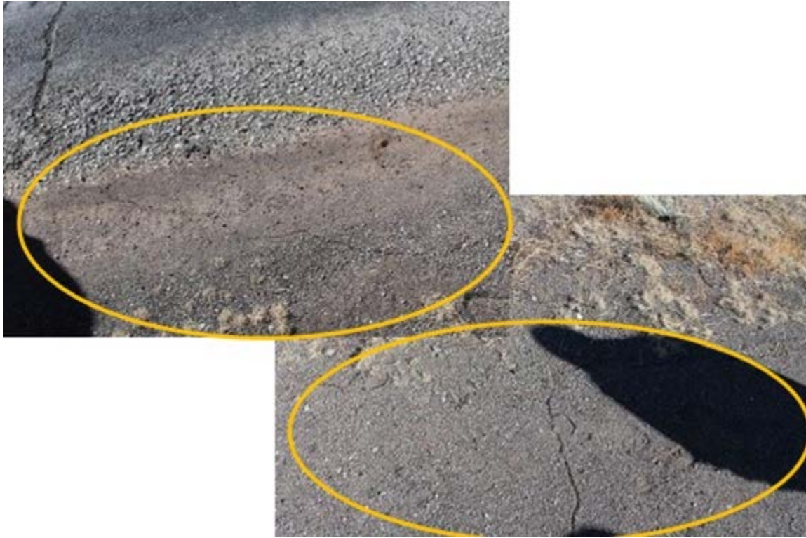
FIGURE 46 Expansive Clay Found on the Outside Westbound Shoulder.
