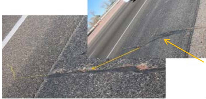
(a) Transverse Reflection Cracking on the Edge of OGFC
