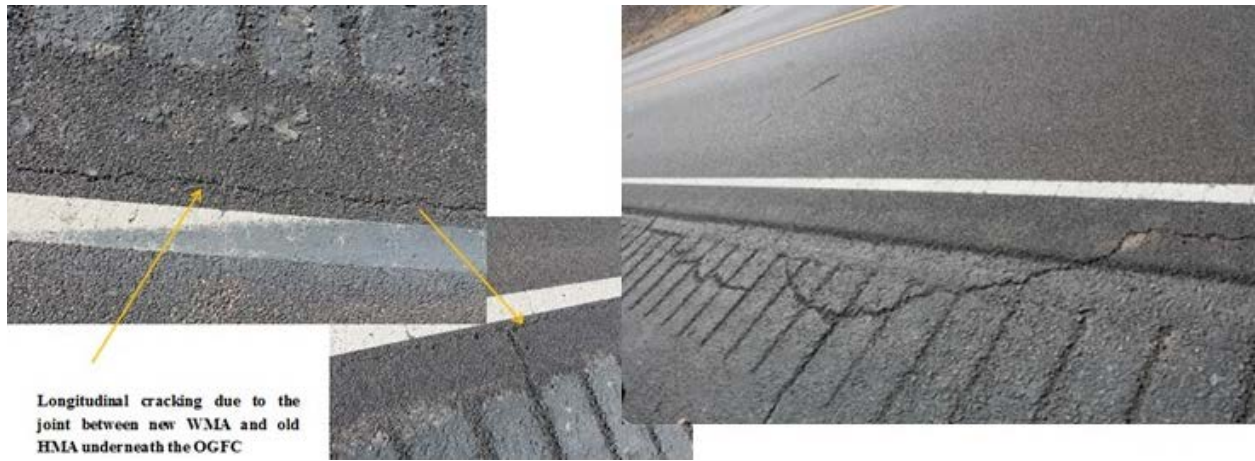
FIGURE 44 Longitudinal Cracking on the Edge of OCFC and the Existing HMA Shoulder.
