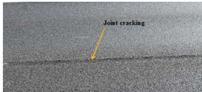
(b) Normal Joint Cracking
