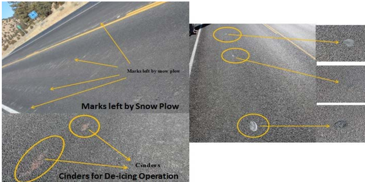
FIGURE 30 White Marks and Cinders (Left) and Binder Balls (Right).
