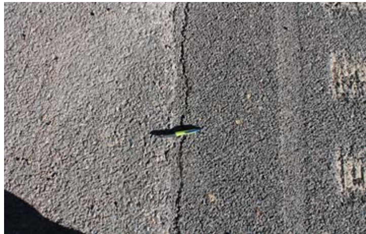
(a) Reflective Cracking along the Edge of Pavement
