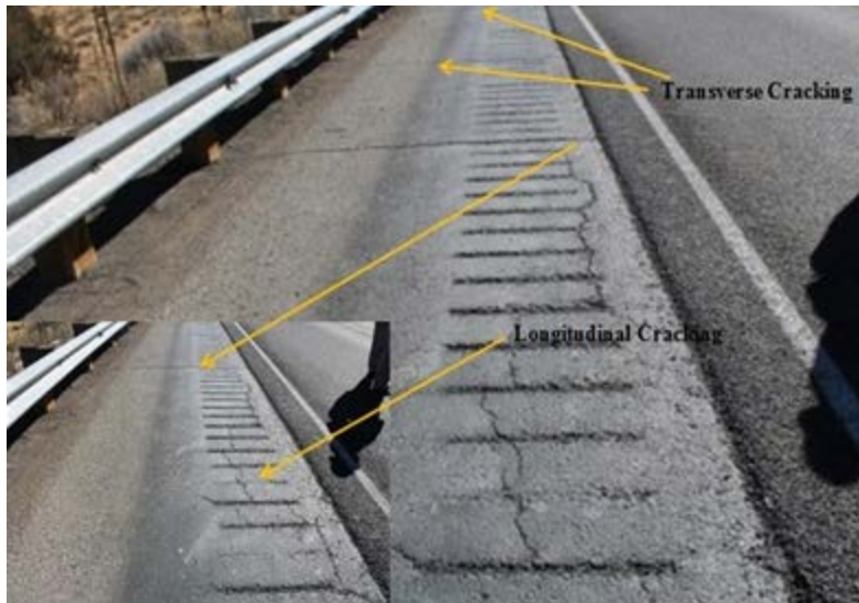
FIGURE 32 Longitudinal Cracking on Shoulders.
