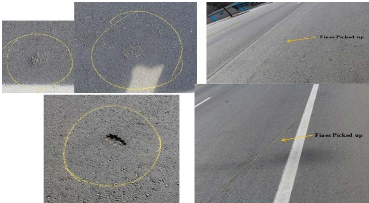
FIGURE 35 Pitting (Left) and Fines Picked Up (Right).
