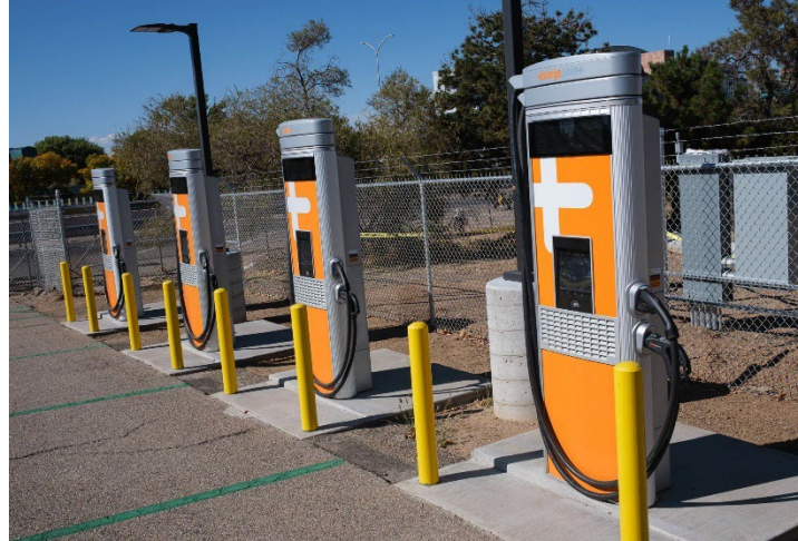
Figure 5. Electric Vehicle Charging Stations at NMDOT District 3
