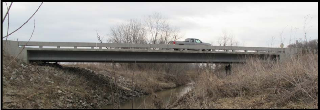
FIGURE 3.1 Mars Hill Bridge: The First UHPC Bridge Constructed in the United States.
